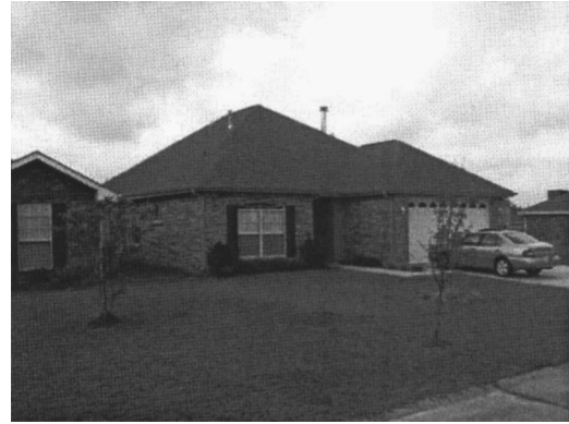
Fig. 22. Example of a hip roof, which performed very well during the hurricane winds
