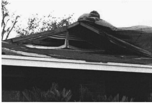
Fig. 20. Attic vent allowed attic to pressurize and roof sheathing to fail
