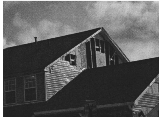
Fig. 10. Loss of nonstructural sheathing at the gable end wall
