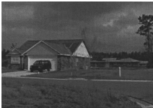
Fig. 21. Newer home with very little structural or nonstructural damage in the foreground; older neighborhood in the back ground with most structures having significant damage
