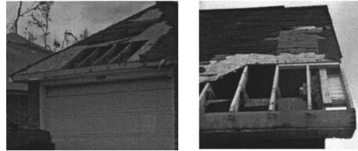
Fig. 9. Roof sheathing damage; a heavier nailing schedule may help protect against this type of damage
