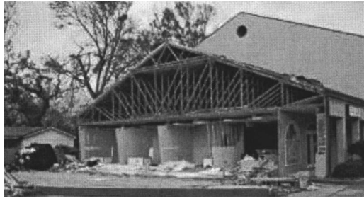
Fig. 7. Loss of CMU wall that was not properly connected to the structure
