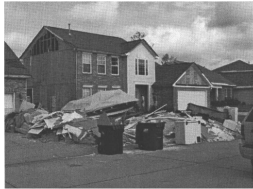
Fig. 18. The result of vinyl siding and nonstructural sheathing loss left just a shell for many of the homes in this subdivision
