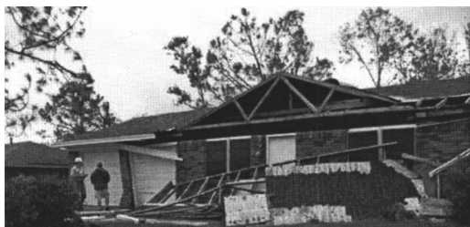
Fig. 4. Porch overhang collapse due to lack of anchorage for support column/post
