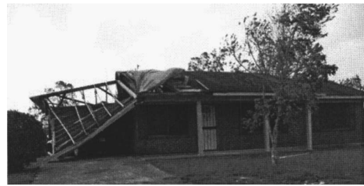
Fig. 5. Carport collapsed and structure breeched
