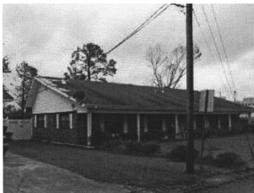
Fig. 17. Loss of roof shingles on an older home; this was quite common for regular roofing shingles
