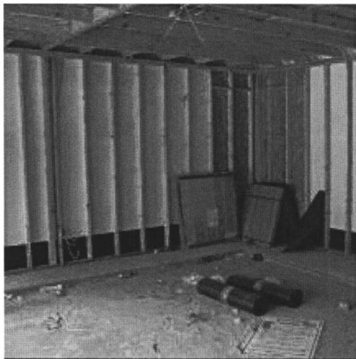
Fig. 13. Braced-wall panels (prescriptive) at the ends of an exterior wall in a region having a design wind speed of 130–140 mph
