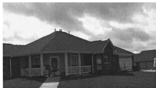
Fig. 19. Damage to the top right trim piece on the roof just left of the garage; this was the only damage to this one-story house with a hip roof
