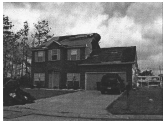
Fig. 11. Loss of gable end wall, roof shingles and sheathing, and garage door (note the debris bags to the left of the driveway)
