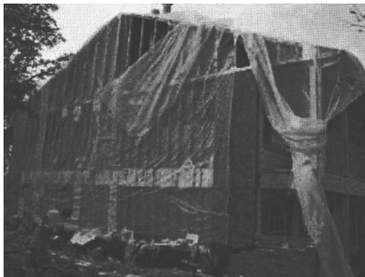
Fig. 8. Loss of brick veneer due to lack of anchorage
