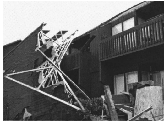
Fig. 14. Condominium roof, retrofitted onto the original flat roof, failed after approximately 4 h of wind gusting
