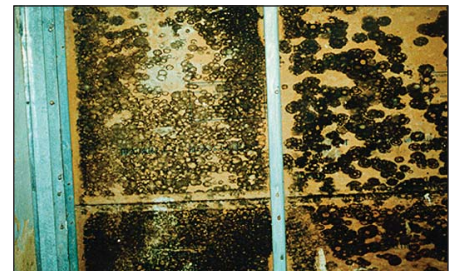
Rising damp. Mold, growing here in a flooded school basement, can worsen asthma.
